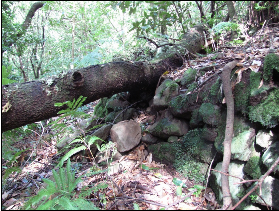
Figure 36: Damaged dry-stone wall due to a fallen trunk, Fajã Fernandes, São Vicente
