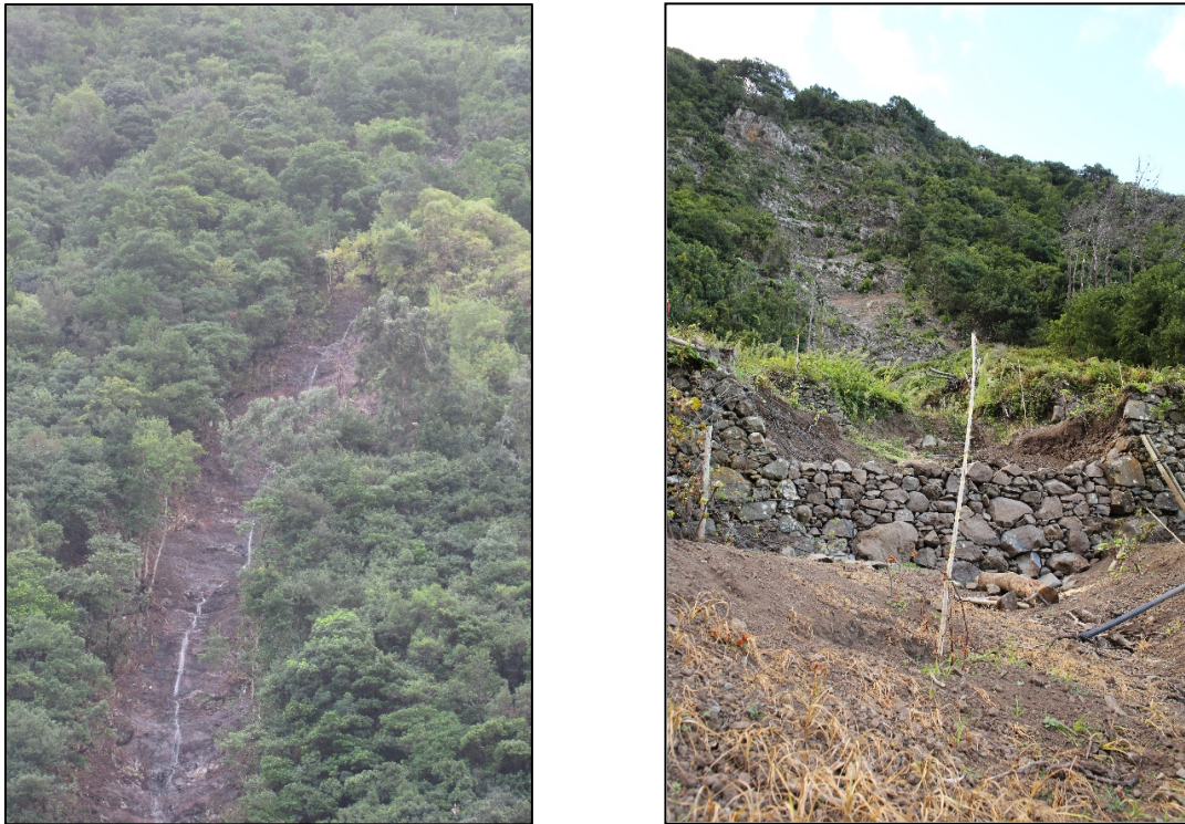
Figure 53: Landslide damage above and within agricultural areas, image on the right by Bork, 2013
